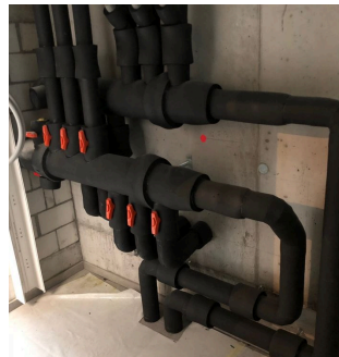
Plant room: manifolds of the external circuits
